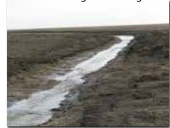
Lateral ditch that requires proper sloping and grass seeding to revegetate.
