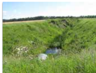
Slumping along the ditch. Erosion control maintenance needed.
