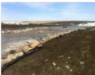
More geo-tech fabric and rock needed to be added to the sides of the ditch.
