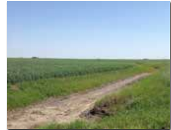
Lateral drainage ditch that requires additional grass seeding.
